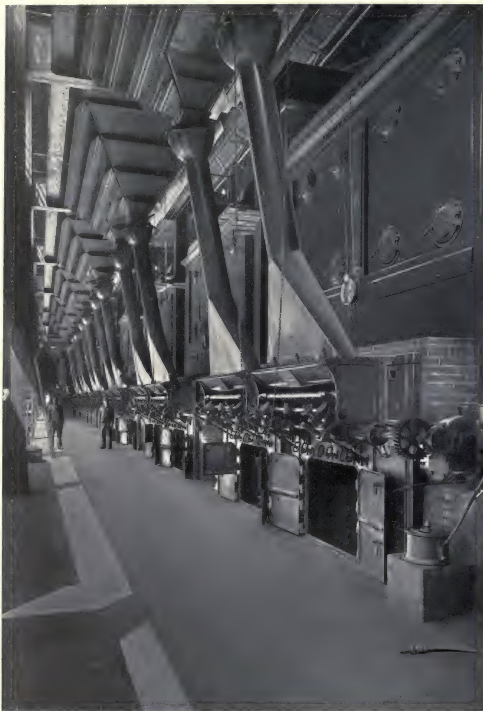
REPUBLIC IRON & STEEL CO., YOUNGSTOWN, OHIO. OPEN HEARTH PLANT 6000 HORSE-POWER INSTALLATION OF STIRLING BOILERS, EQUIPPED WITH BABCOCK & WILCOX SUPERHEATERS
